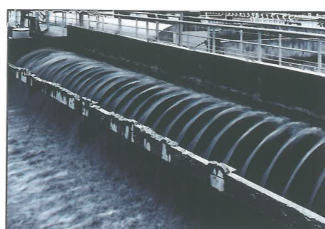
Disinfection of industrial water pretreatment
